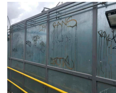
More graffiti. The bridge is a mess.
