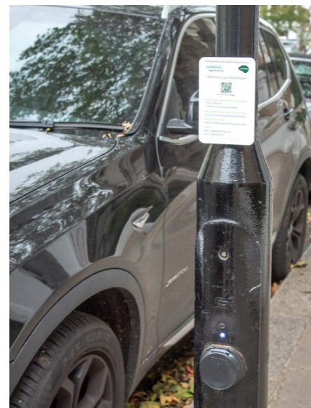
Fighting climate change. An increasing number of EV charging points are being installed in Westminster.
