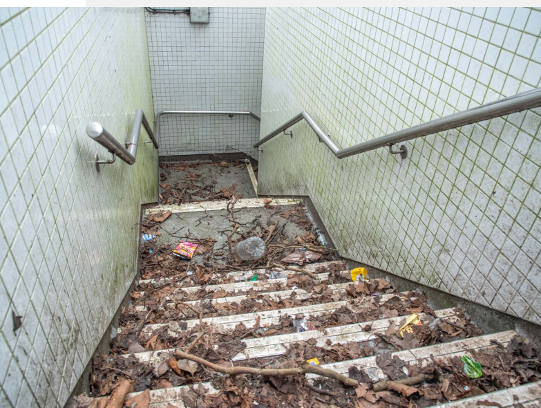
The stairs to the toilets are still strewn with rubbish.
